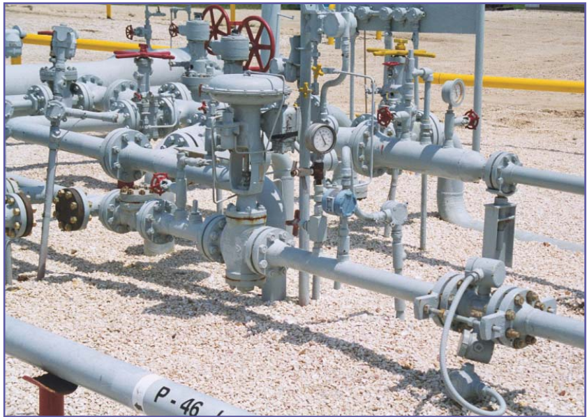
A common meter-run setup.
