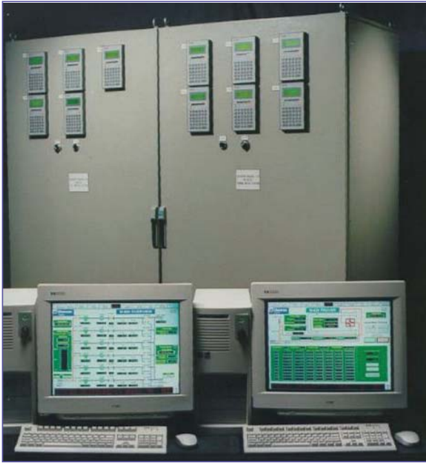
Installation of flow computers communicating to a PLC system within a control room environment.
